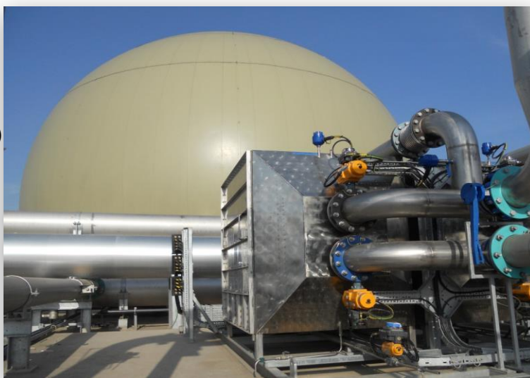
BioGas BGAK on WwTW site.
